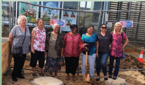
Turning the first sod for construction of the Rainbow Serpent water feature
